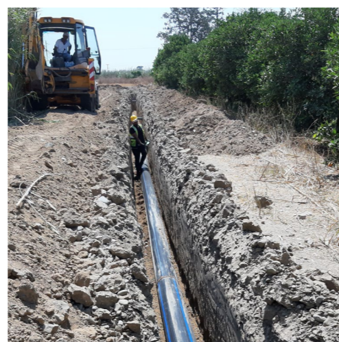
High-density polyethylene (HDPE) water distribution pipes of the kind shown above have now replaced the old pipes
